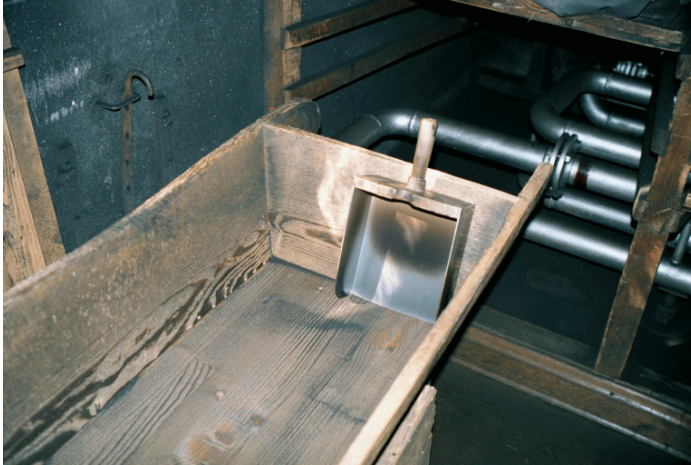
Figure 34. Steam pipes that heat air under the racks. The photo on the left shows the steam pipes running beneath the drying racks that heat air to dry the powder spread out on the drying tray cloth.
