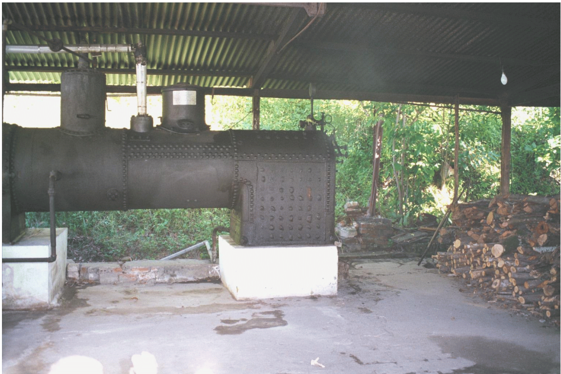
Figure 22. Wood fired boiler used to generate steam for the drying house.
