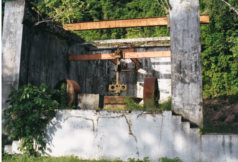
Figure 5. Wheel mill destroyed by fire/explosion in 1995.
