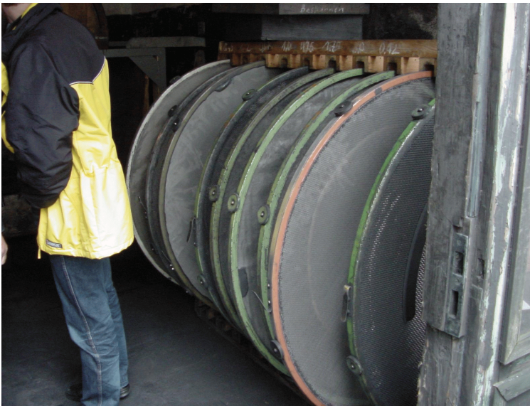
Figure 71. Screens at WANO in Germany.
