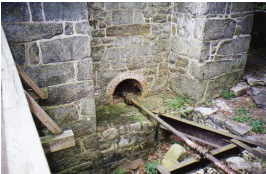
Figure 31. Drive shaft from turbine.
