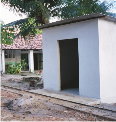
Figure 20. Mill batch storage
