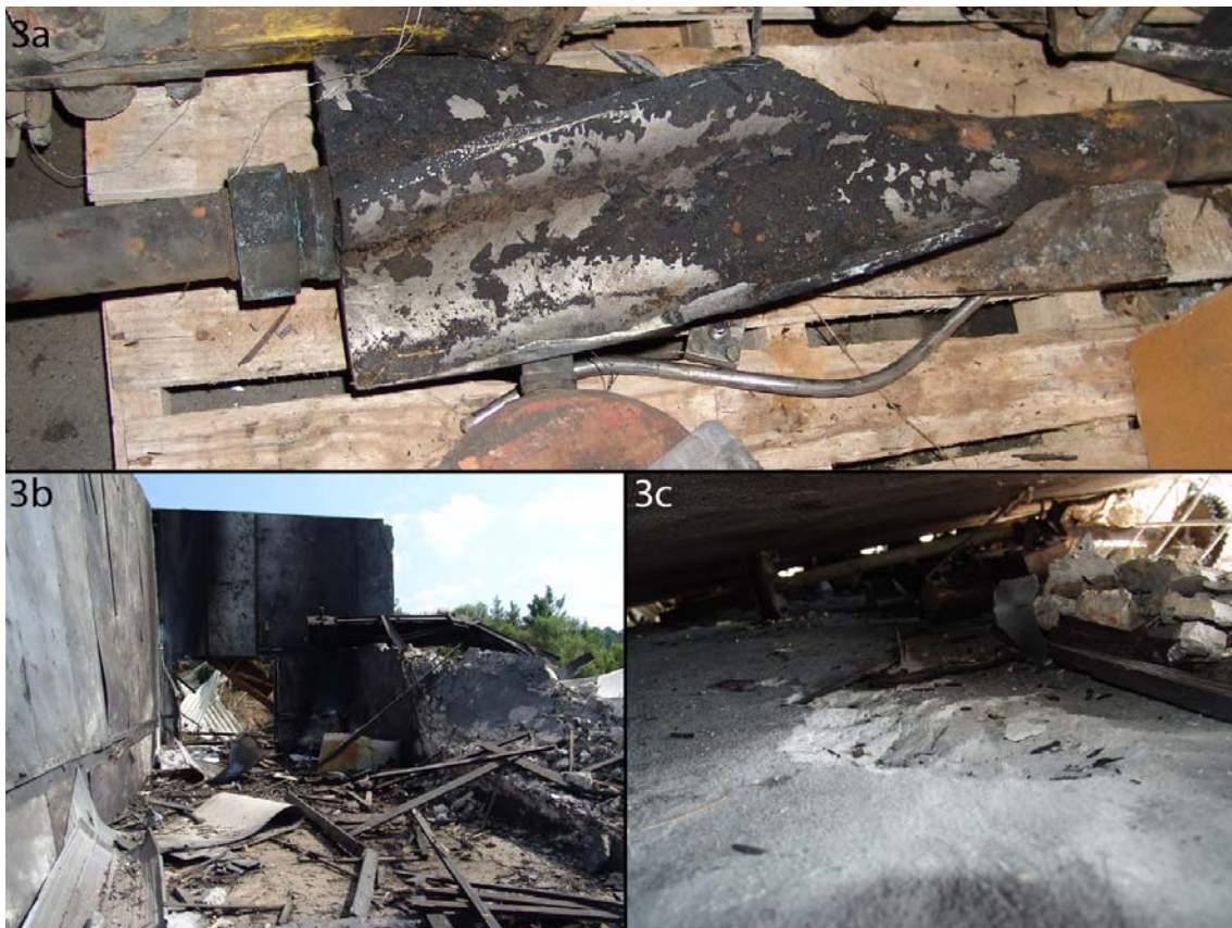
Figure 3: Fragmented worm (a), destroyed corning mill (b) and crater under hopper and worm (c)
